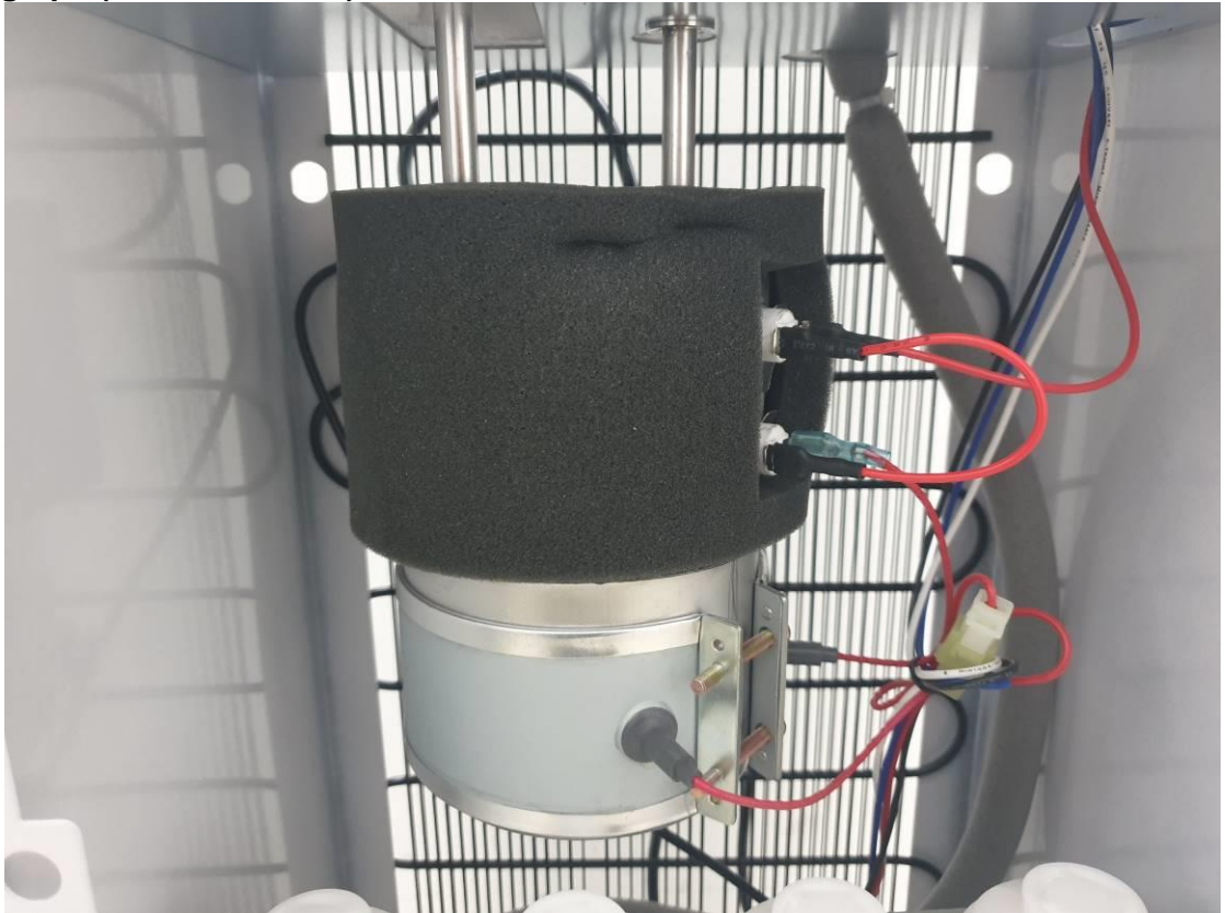
<Hot water tank>
