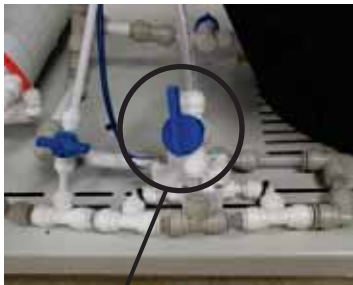
Pressure Tank Drain Valve
